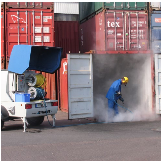
Reinigung eines Containers Container cleaning Nettoyage de conteneur
