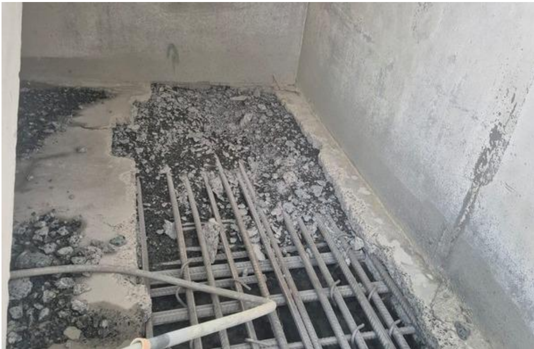
Figure 1 — Aqua Cutter 410V Hydro Demolition Robot operating on site beneath the stair landing
